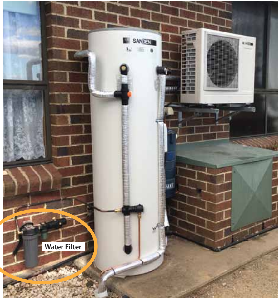
Typical water filter installed
