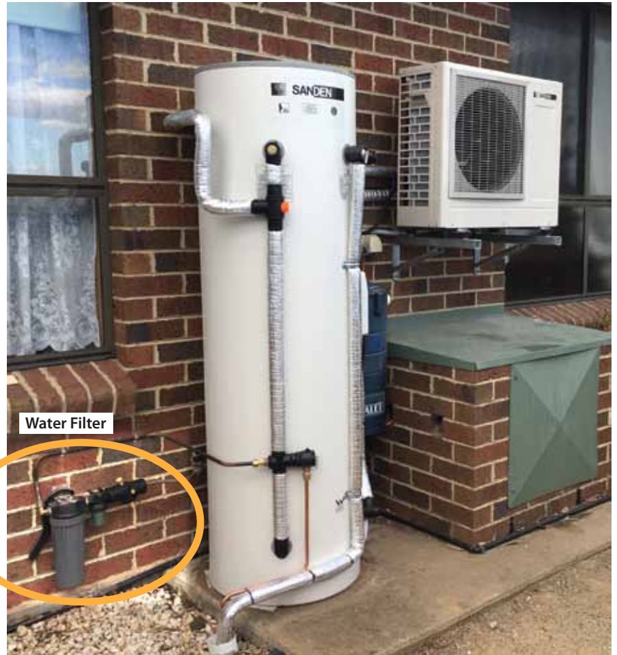
Typical water filter installed
